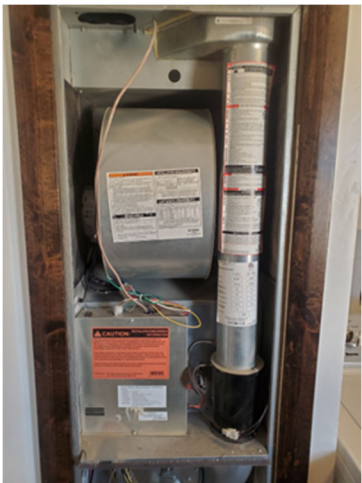
Furnace in House
