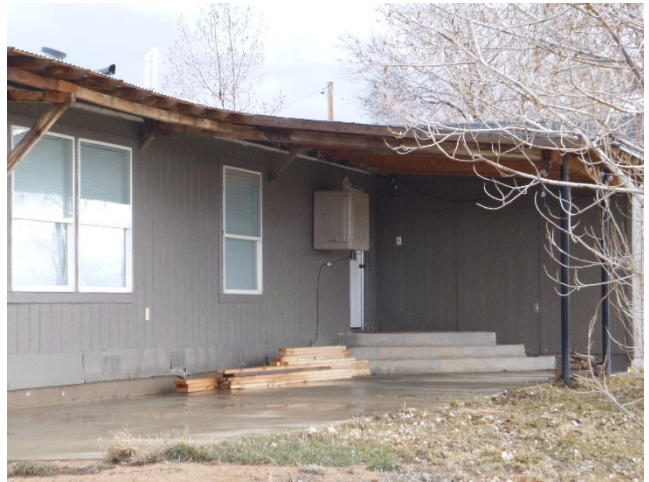
Swamp cooler at house
