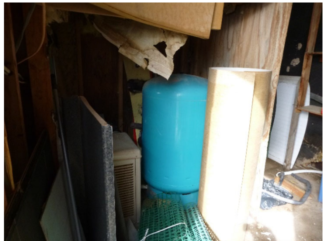
AC Tank in outbuilding
