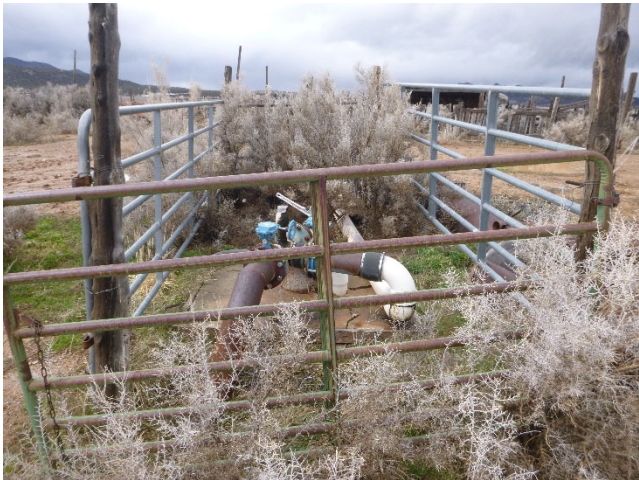
Pump (looking west)
