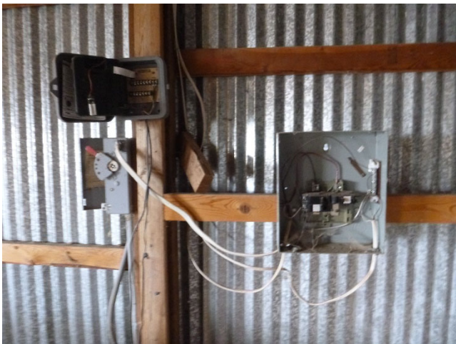
Electrical box inside unfinished housing unit
