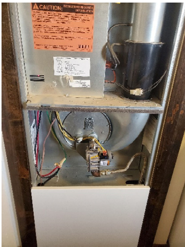
Furnace in House
