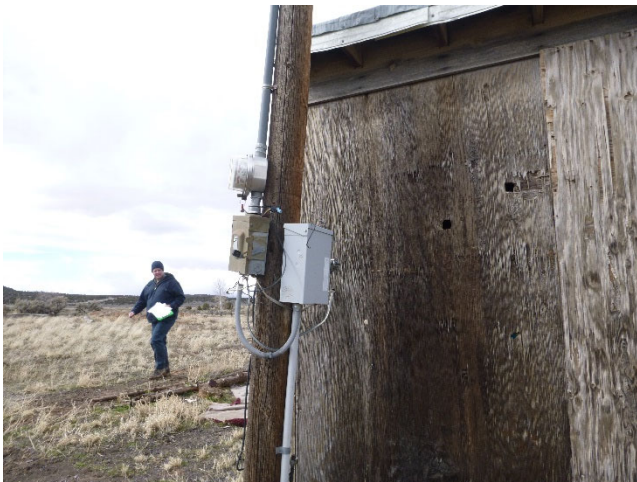
Electrical box on outbuilding
