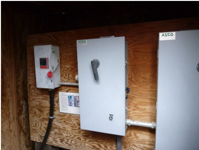
Well Control Box
