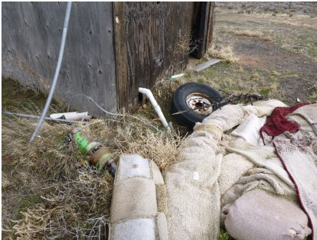
Septic system location (believed) outside outbuilding
