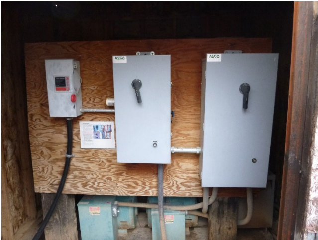
Well Control Box
