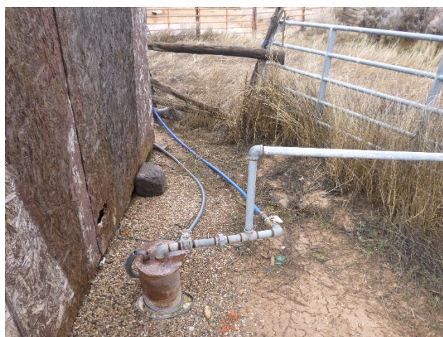
Pump (looking west)
