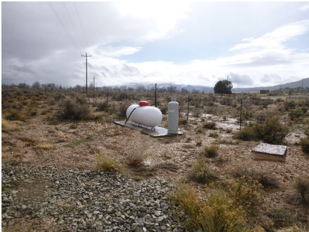
Propane tank (looking SW)
